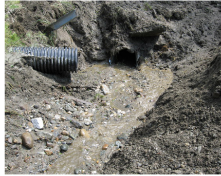
Stockbridge culvert before it was repaired with Better Roads funding | © TRORC Staff
