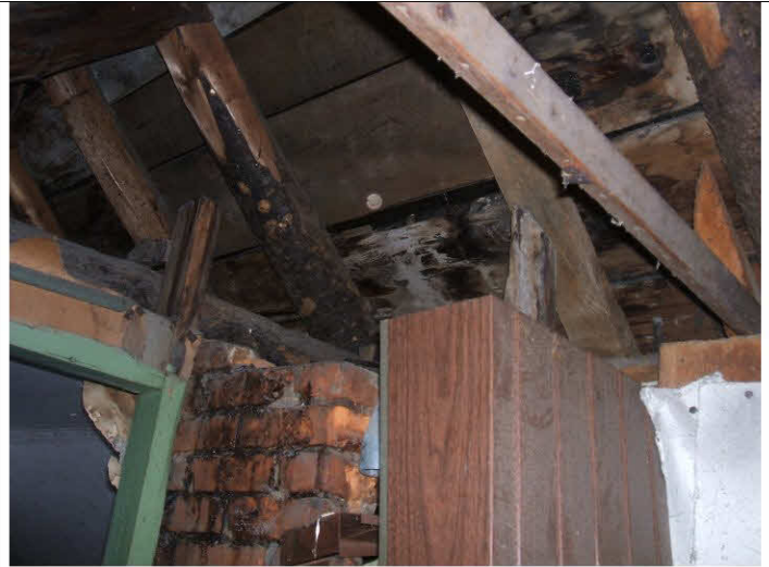
The top of a defunct chimney in the attic. It has a plug in it but I am not sure that it is air sealed.
