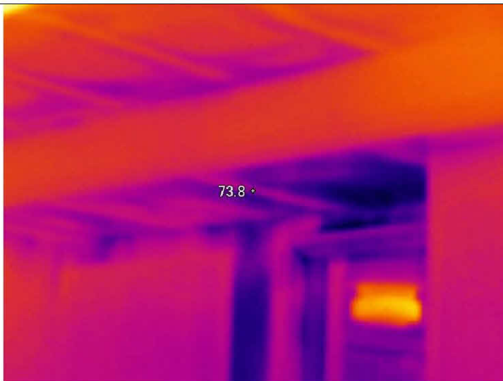
Cold ceiling bays and interior wall bays where the ceiling changes plane.
