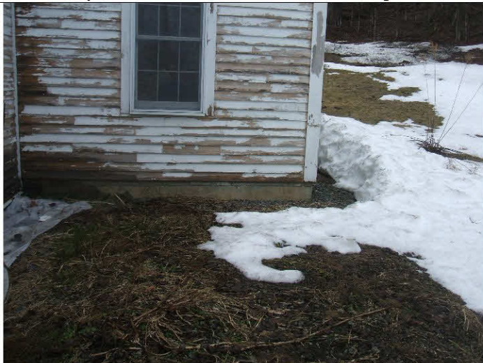
The clapboards are in need of repair and paint.
