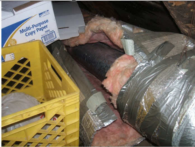
The existing ducts are poorly sealed and insulated.
