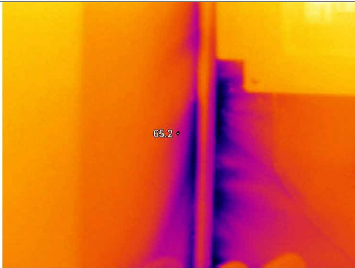
Air leakage in the corner of the boiler room.
