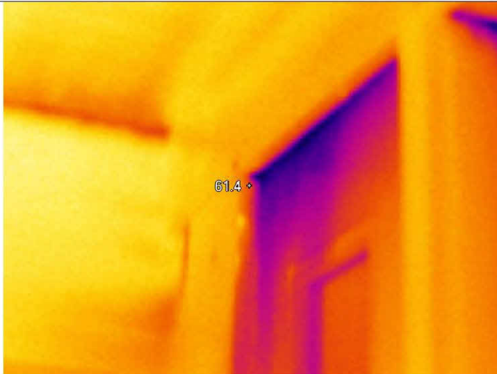
Air leakage around the door side light.
