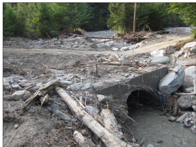
Photo 4: Severely Damaged Culvert, Stockbridge Photo Source: Chris Sargent
