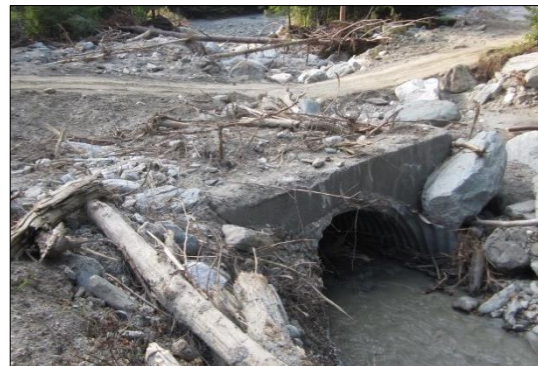
Photo 4: Severely Damaged Culvert, Stockbridge Photo Source: Chris Sargent
