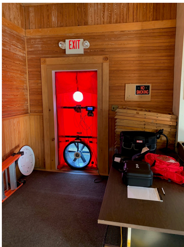
A "blower door" air leakage test underway in Topsham's Town Hall. | Photo: Harry Falconer, TRORC Staff
