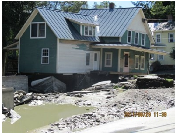
Substantial flood damage to a residence in Rochester following TS Irene. Photo: Toby Talbot, Associated Press
