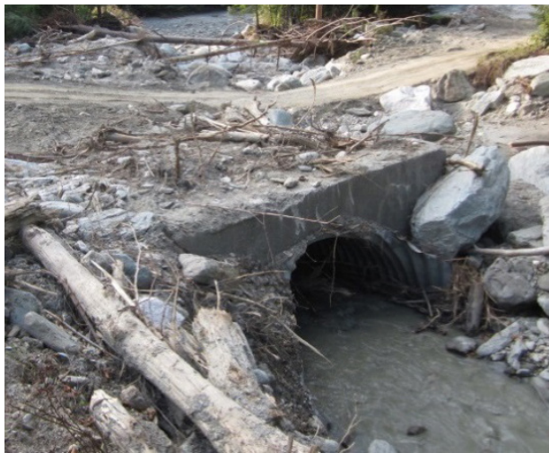
Severely Damaged Culvert, Stockbridge | Source: Chris Sargent
